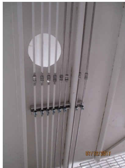
Figure 10: Example of rigid helium lines on a VLA antenna.
