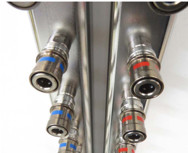
Figure 6-6 View looking down the stainless-steel manifold, located at the rear of the rack. The manifold provides the interface between the cold plate attached to the FPGA (etc.) and the CHx40 heat exchanger. The manifold has a supply and return side, providing 2 hoses to each TALON-DX board (i.e. 4 per LRU).
